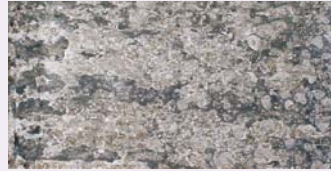
Where corrosion is already evident, ACF-50 will inhibit further progress stopping the corrosion process on contact.
